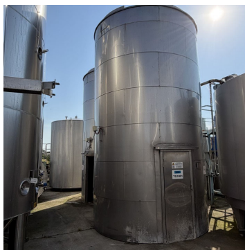
2 cuves inox 25426 litres CSC – calorifuge S/S insulated tanks
